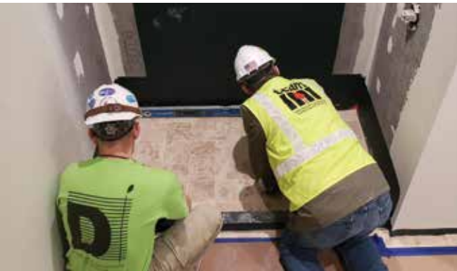
Fig 3. Tile in areas that are soaked, saturated, or regularly and frequently subjected to moisture, like residential showers, should use an installation method having environmental exposure classification of Res3 (Residential Wet) or Com3 (Commercial Wet).
